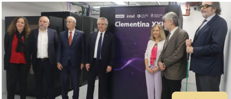
In October 2023, Prof. Saulo, in her role as director of the SMN, and colleagues kicked off construction of Clementina XXI, a new super-computer for SMN
